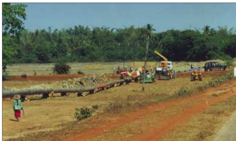
A gas pipeline is being connected between Kaunbawk and Myiang Kalya in Mon State.
