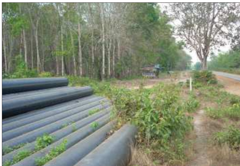
New pipe segments are seen stacked in a pile with a guard shack for villagers to guard seen in the background near Waekhami village, Thanbyuzayat Township early in 2011.
