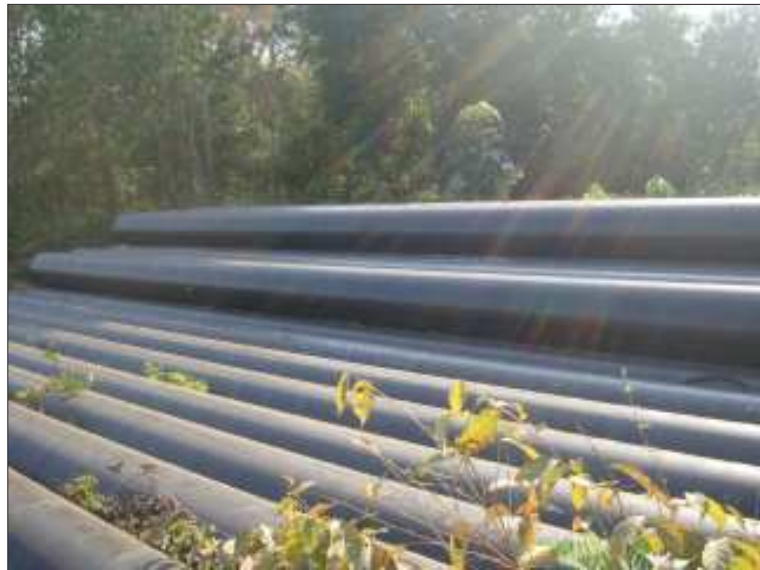
Pipeline segments are seen stacked in a pile near Kaungywa village, Thanbyuzayat Township prior to construction.
