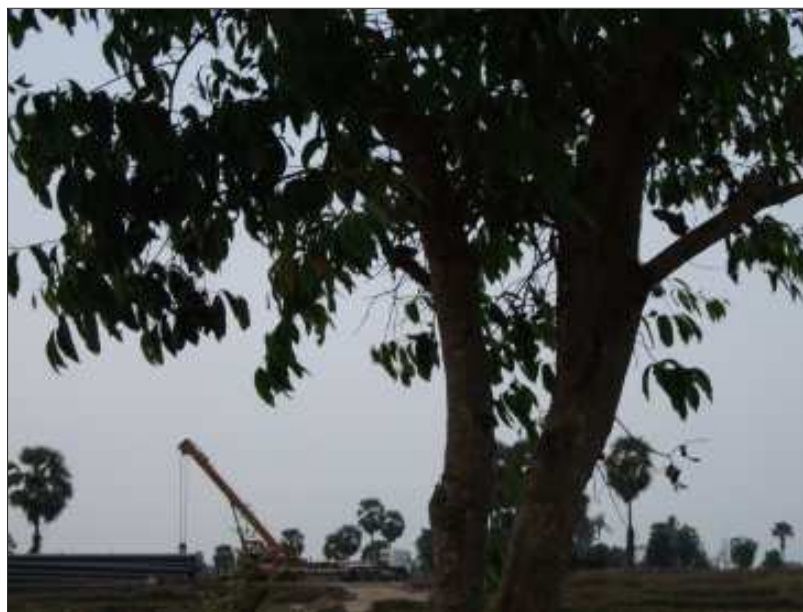
A crane belonging to MOGE is seen installing new pipes on the Kanbawk to Myaing Kalay near Lamine sub-township.
