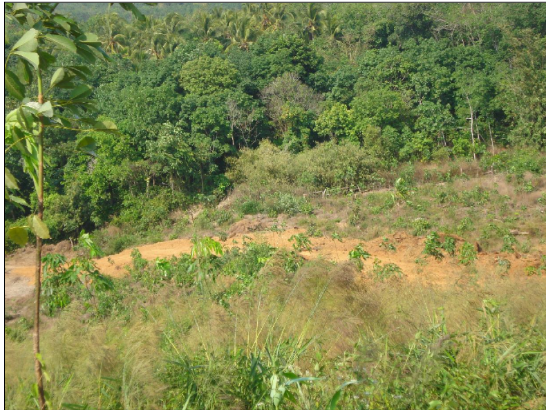
A section of the new road which damaged 2 acres of a 4 year old rubber farm, is seen near Sintaung village, Thanbyuzayat township, Mon State.
